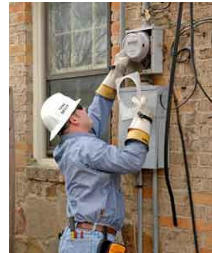
Natural Gas Leaks
